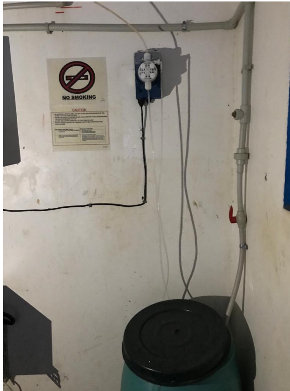
Figure 8.3: Automatic chlorine dosing at the Buwuni reservoir
