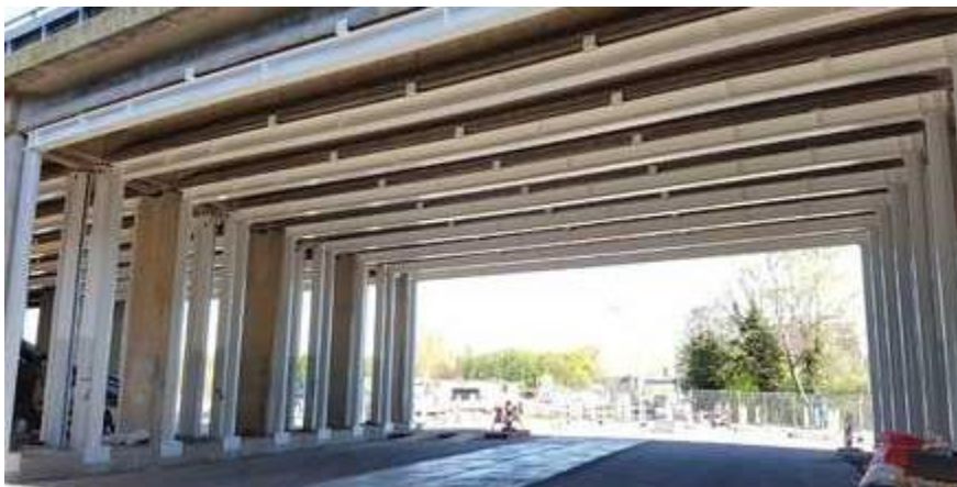
Figure 7.7: External steel support structure A4 Ringvaartviaduct (Mourik, 2019)
