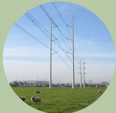
Figure 31: Wintrack transmission tower
