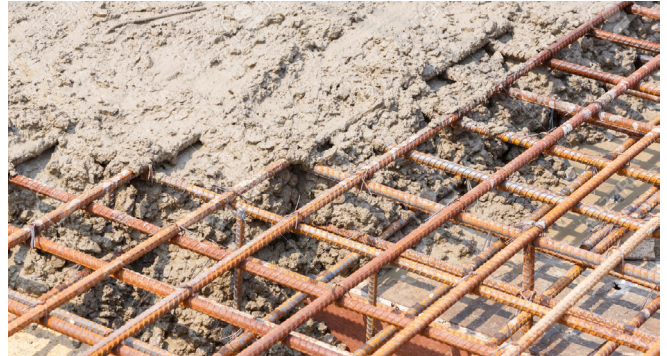
Figure 4: In reinforced concrete, steel bars are the dispersed phase and a cement mix is the matrix.
