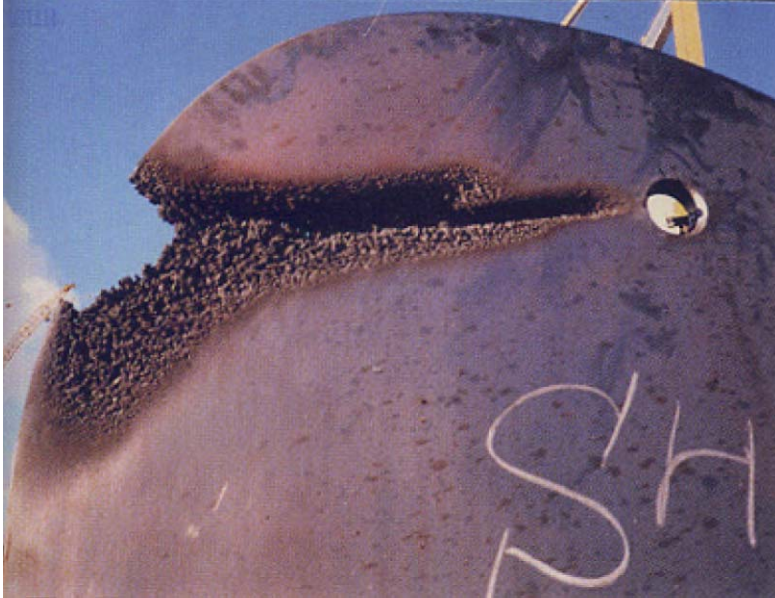
Figure A-4: Cavitation damage due to missing plug
