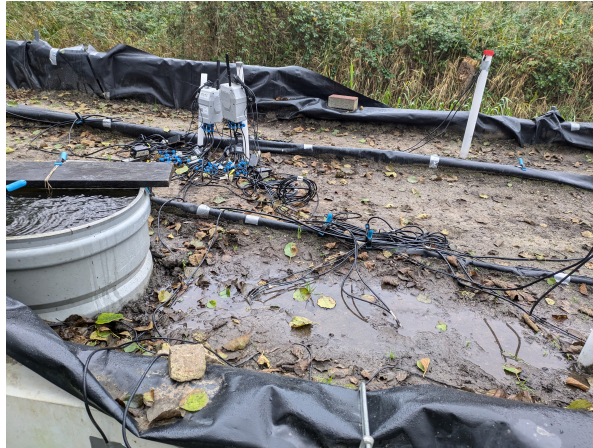
Figure 3.6: Pooling above sensor profiles during tracer testing in swale #1.
