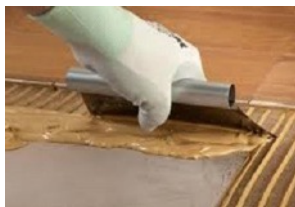
Figure 47 – Adhesives and sealants and other liquid bonding methods are regularly used in construction. But how can this floor be reused when it cannot come off undamaged?
