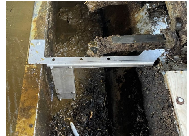
Figure 51 - Sensor mounted inside the Sphere siphon
