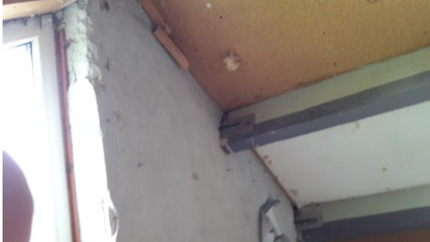
Figure 7: View of Z2 roof panels and purlins (the white-coloured part is only a piece of wall paper).
