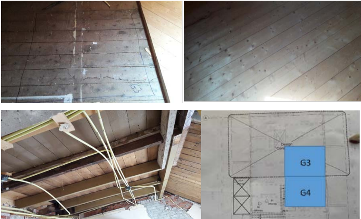
Figure 5: Floor samples G3 and G4; upward and downward facings and location in the house.
