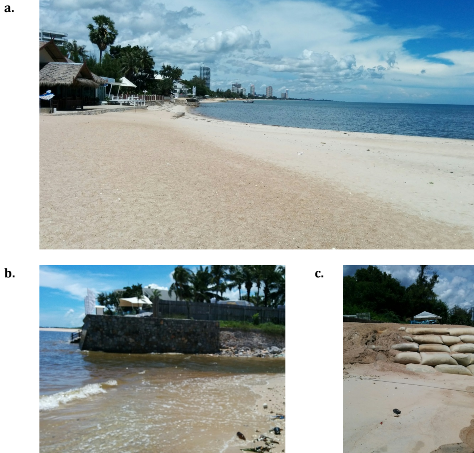
Figure 2.2 | Problems at Cha-am. (a) Beach north of the offshore breakwaters, below in the picture the beach is wider due to a recent nourishment. (b) Farther away it is visible that the beach has completely eroded away. (c) Even further away there are exposed sandbags. These sandbags were placed as part of a recent nourishment, the sand layer covering them has been completely eroded already (own pictures).
