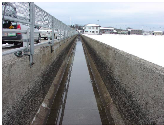
(a) Before Repair
