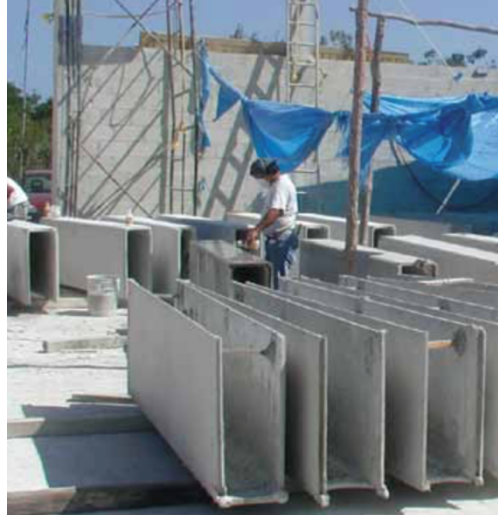
Figure 108 GFRC permanent formwork for beams in Puerto Rico. Courtesy of Nippon Electric Glass America Inc (Banthia et al. , 2012).
