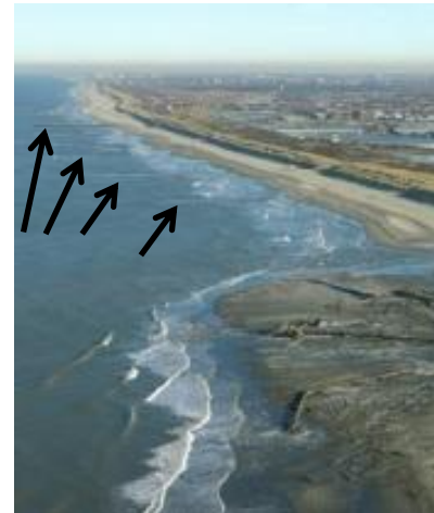
Figure 3: Aerial photograph of the northern end of the Vlughtenburg field site during construction. Groynes at the southern end are already covered with sand. (source: www.delflandsekust.nl )
