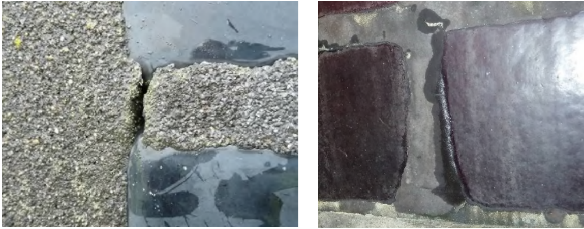
Figure 2.3: Visible cracks in the epoxy mortar and de-bonding of the glass-resin interface simultaneously with moisture ingress [4].
