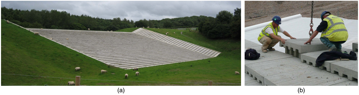
Fig. 1. Prototype stepped spillways with inclined downward steps for Bruton flood storage reservoir, UK ( \theta = 14^\circ , H = 10.75 m, B = 48 m, and Q \approx 250 m 3 /s): (a) general view of the spillway shortly after completion in 2008; and (b) construction details with installation of precast concrete blocks over the geotextile membrane. (Images courtesy of John Ackers.)
