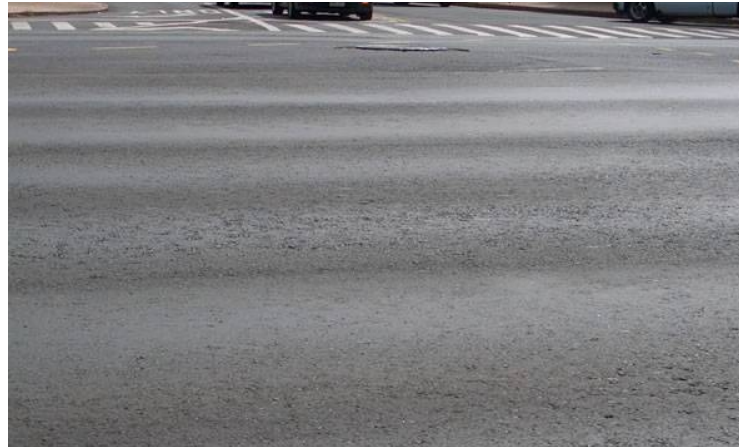
Figure 2.8. Rutting of dense asphalt concrete (after Muench, 2003).
