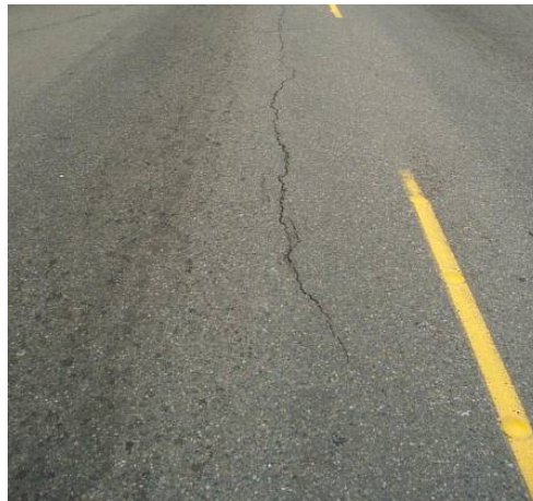
Figure 2.6. Longitudinal cracking of dense asphalt concrete (after AWV, 2001).
