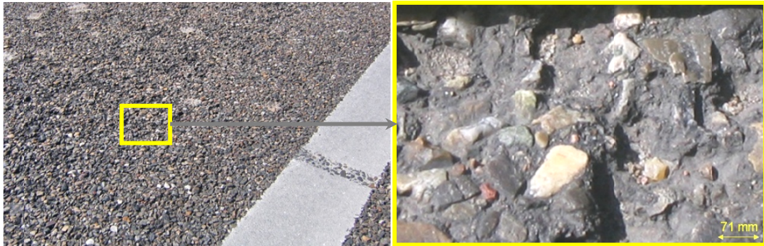
Figure 2.3. Raveling of porous asphalt concrete (left) means that the pavement surface loses aggregate particles (right).
