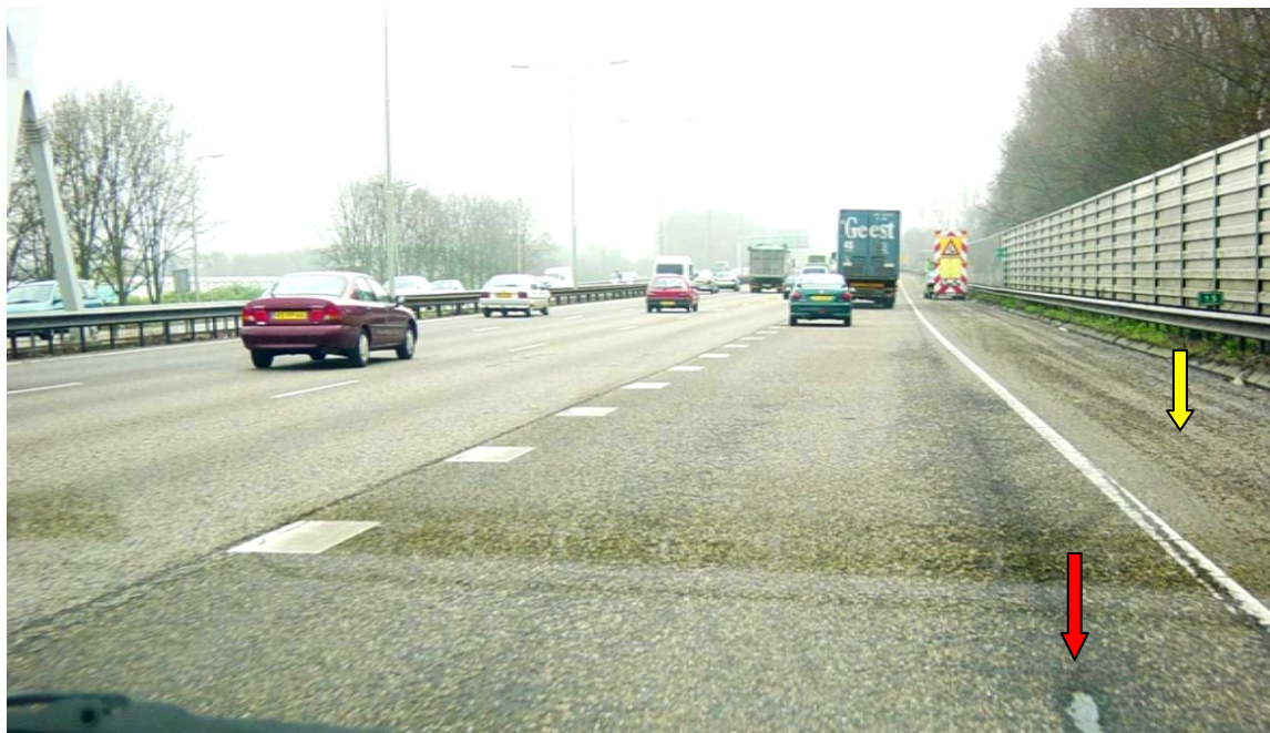
Figure 2.4. Raveling of porous asphalt concrete on a Dutch motorway.
