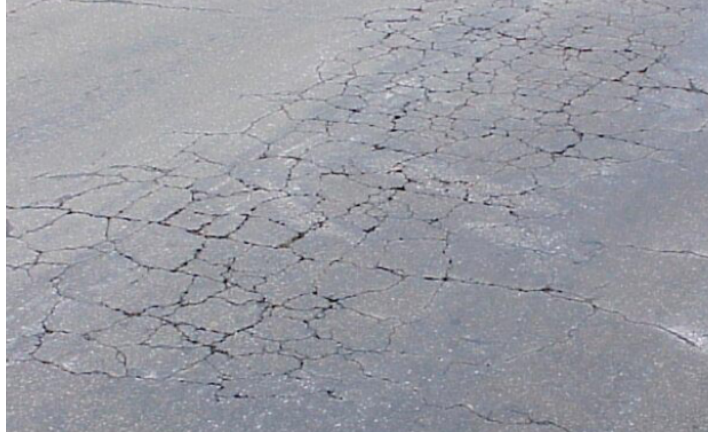
Figure 2.7. Alligator cracking of dense asphalt concrete (after AWW, 2001).
