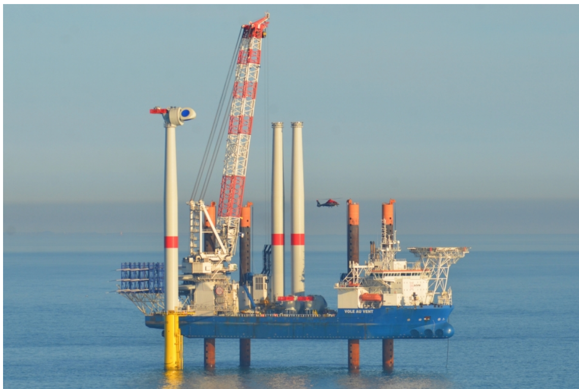
Figure 1.1: Jack-up vessel in elevated condition during offshore wind turbine installation (SWZ Maritime, 2022)
