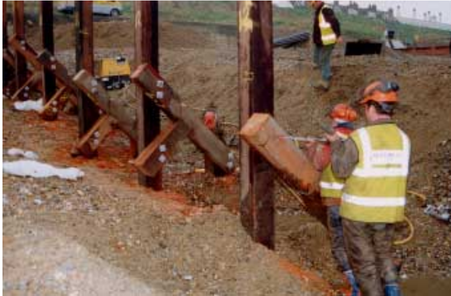
Figure 35. Y-shaped raking struts (courtesy to HR Wallingford)
