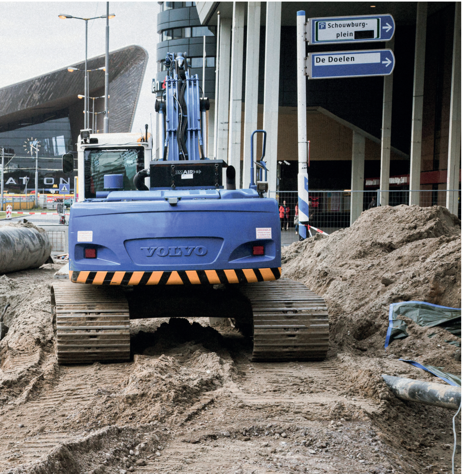
Figure 02: Urban excavation works near Rotterdam Central Station, illustrating soil flows generated by inner-city construction activities. Adapted from Chris Mueller, iStock.com/Chris Mueller, Stock photo ID 45830017, editorial licence.
