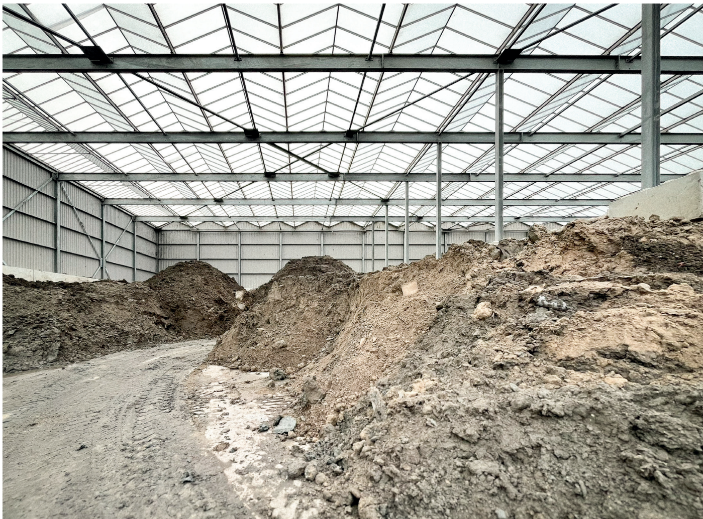
Figure 06: Stockpiled excavation material from trench digging and pipeline installation works in Rotterdam and Delft.
