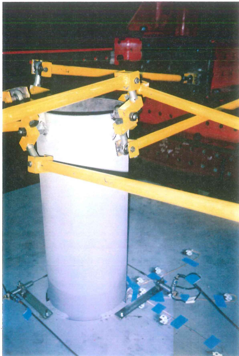
Photo 4-35 : Instrumentation on 3C2 and lateral supports to column
