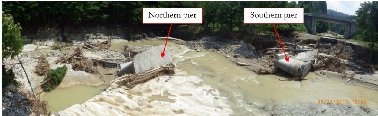
Figure 2: Panoramic photo of the destroyed bridge (taken by J.D. Bricker, 2013)
