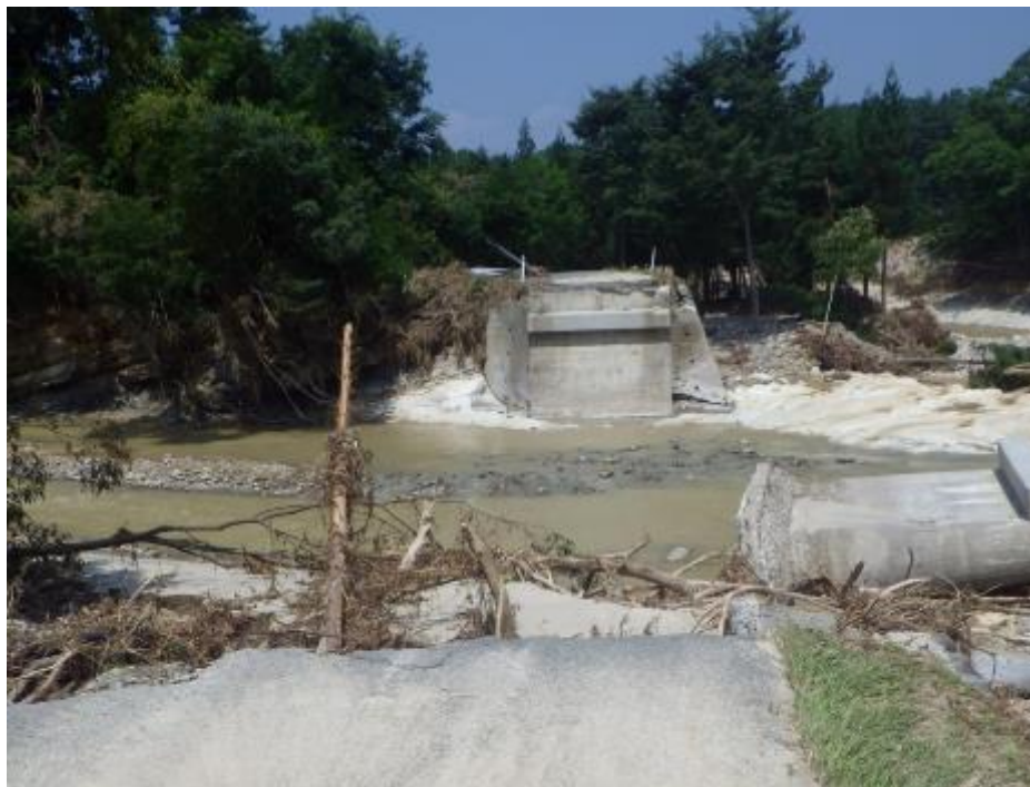
Figure 1: Photo of destroyed bridge crossing Yabechi River (taken by J.D. Bricker, 2013)
