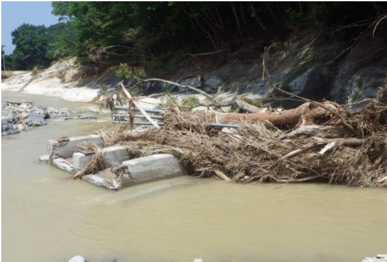
Figure 3: Photo of one of the dislodged deck segments and debris (taken by J.D. Bricker, 2013)
