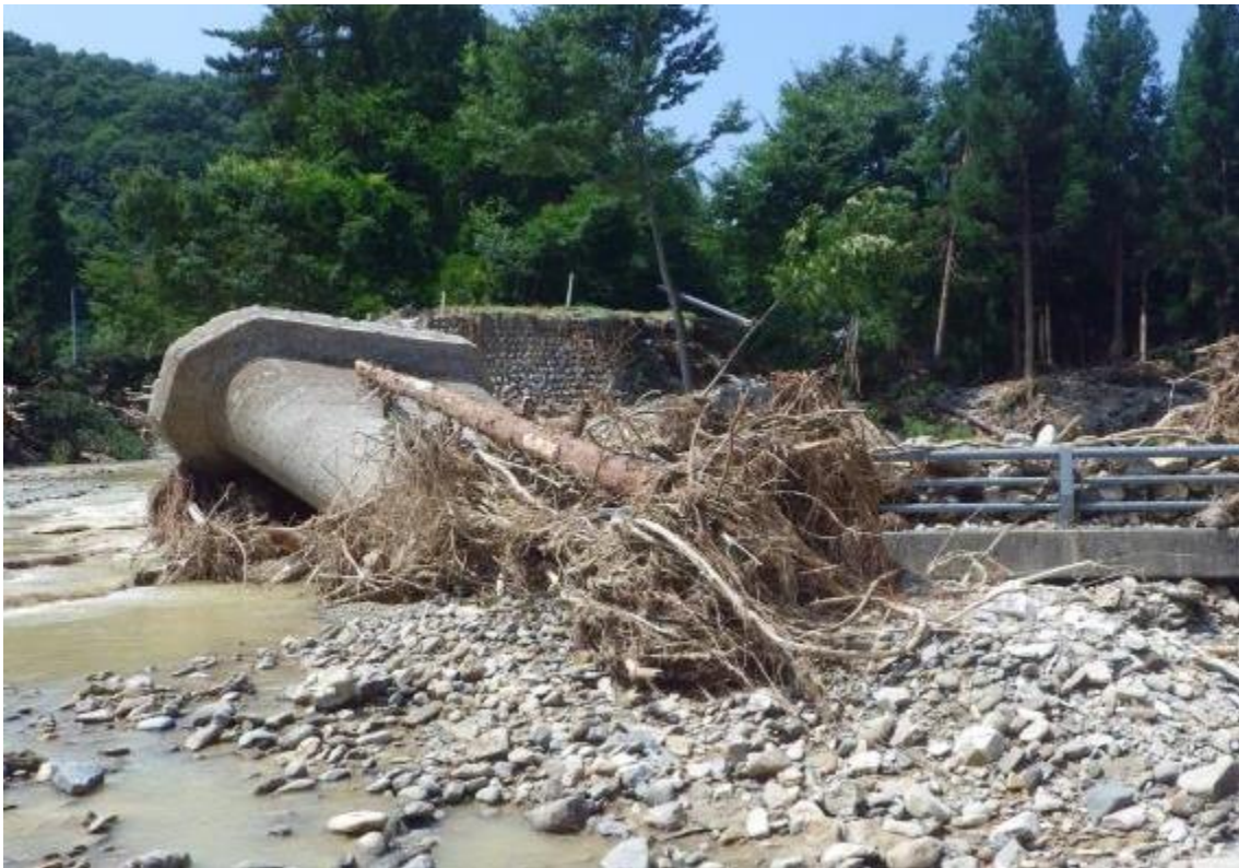
Figure 5: Photo of the collapsed northern pier (taken by J.D. Bricker, 2013)
