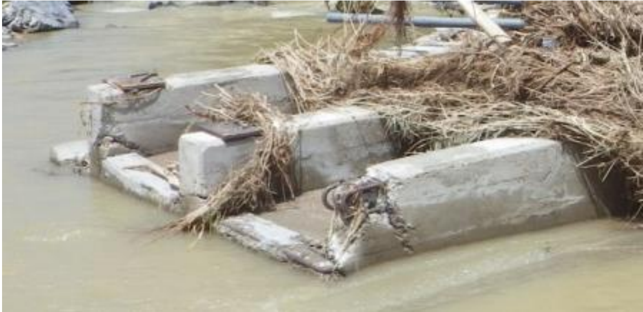
Figure 27: dislodged bridge deck segment showing remains of a bearing
