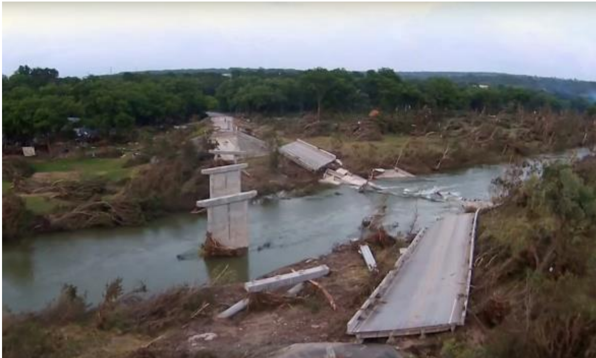
Figure 6: collapse of Fisher Road Bridge over Blanco River at Wimberley, Texas, USA in May 2015 (taken by C. Bailey)
