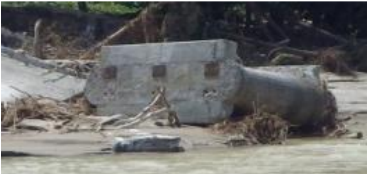
Figure 26: collapsed pier showing remains of a bearing
