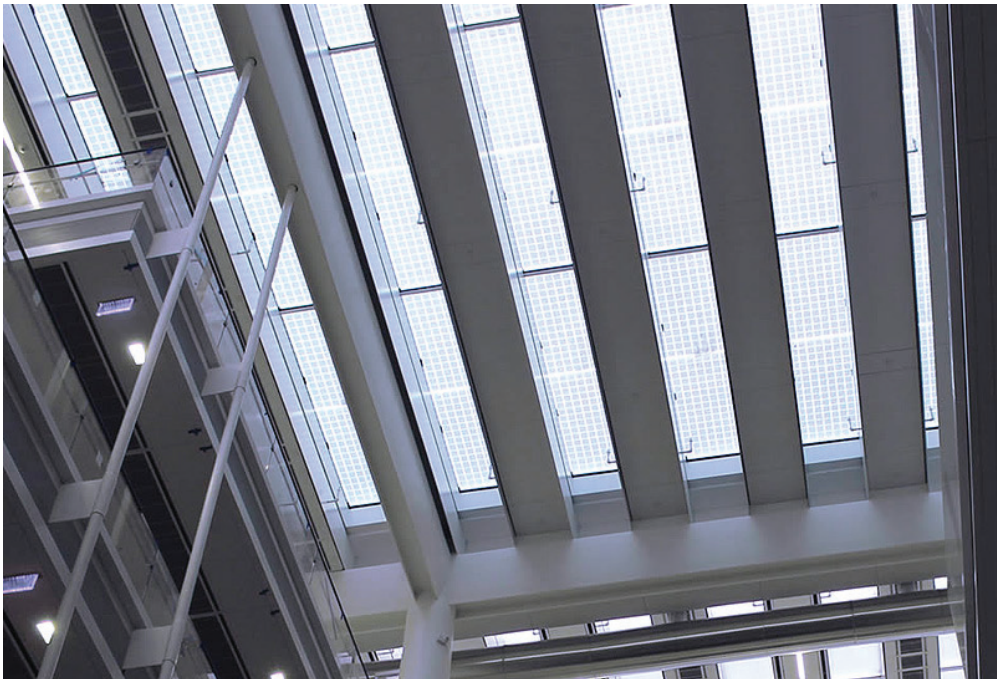
Onyx PV skylight
