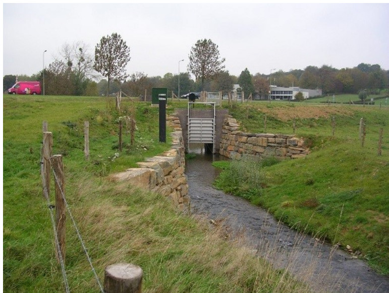
Figure 2.15: The controlled outflow gate of the Buffer Nijswiller in the Selzerbeek (Waterschap Limburg, n.d.-a).
