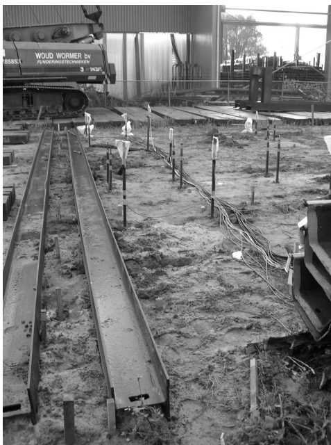
Figure 7.5 Instrumented test site, just before start of installation of the sheet piles
