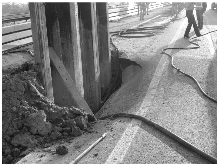
Figure 2.1 Example of excessive settlement during vibratory installation of sheet piles
