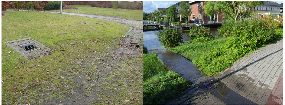
Figure 5-1 Dutch overflow structure to ensure a maximum water depth in swale (left). Overflow of water from swale directly to surface water during full scale testing in Purmerend (right).
