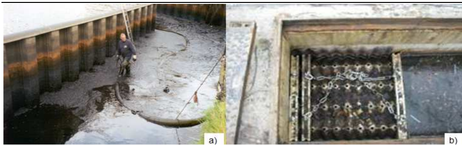
Figure 3-1(a) Sediment basin in Amsterdam (sludge from stormwater system during maintenance after 8 years) and (b) lamella settler in Krimpenerwaard, The Netherlands.
