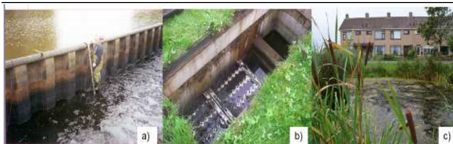
Figure 1-2 (a) Empty sediment basin filled with sludge from a stormwater system after 8 years of operation, (b) sludge from stormwater sewer clogging a lamella settler and c) sedimentation pond
