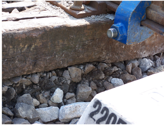
Fig. 1. Severely wore ballast stones under an old sleeper. Compared with the new ballast stones nearby with sharp edges, the wore ballast stones have become rounded in shape and covered by dusts. This problem is called the “foul” of the ballast, meaning that the ballast stones have been crushed, provide less drainage, move less and have less elasticity, leading to a reduction in their friction dissipation.
