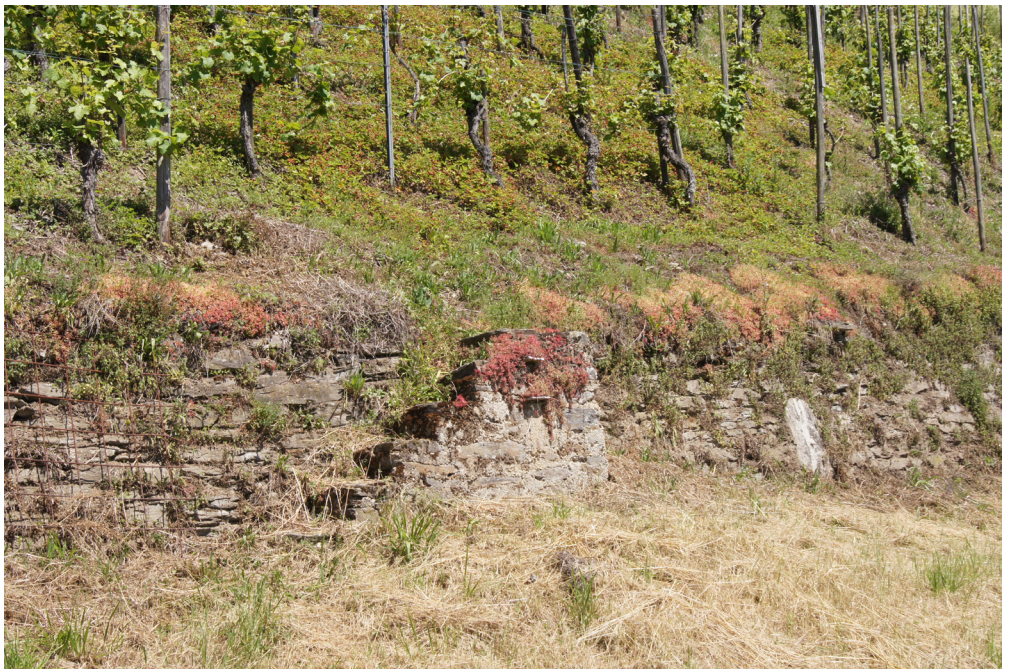
Fig. 44: Drywall overgrown with moss and vegetation.
