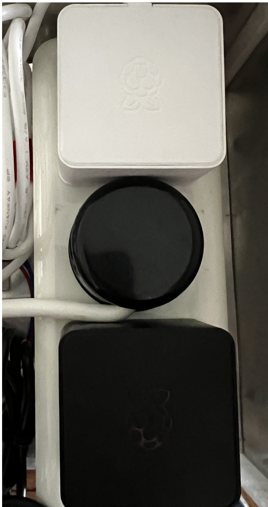
Figure 61: Corrected emergency switch connection and grounding setup inside the PEMAD control unit. The cables are now properly insulated and permanently connected in accordance with the NEN-3140 safety standard. The grounding wire is securely fixed using a standardized grounded plug, minimizing the risk of overheating or short circuits.
