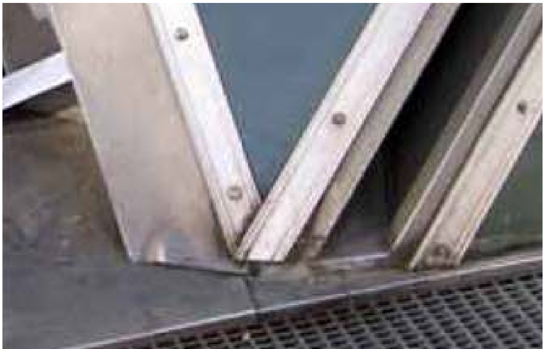
Figure 1.1.5: Non orthogonal façade construction, resulting in a joining detail that is inadequately solved with silicone.
