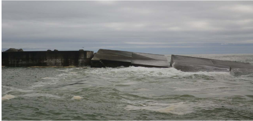
Figure 3.30: Damage of the caisson breakwater (Source: DPRI Kyoto University; Courtesy of Yusuke Tanaka)
