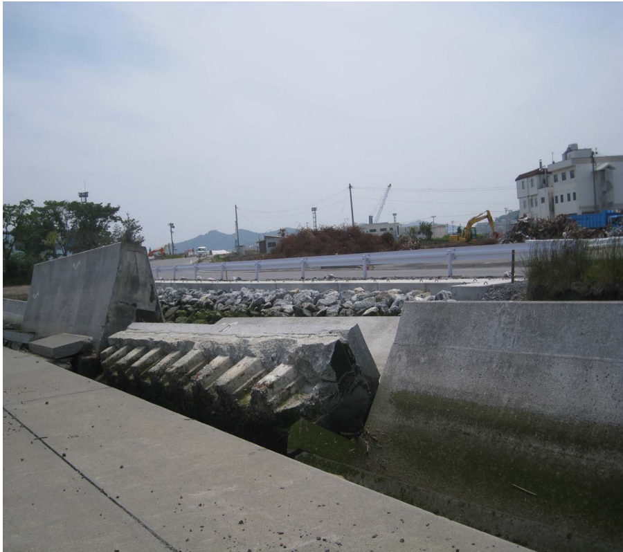
Figure 3.12: Failed sea wall of Ofunato photographed in June 2012.
