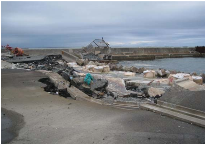
Figure 3.31: Damage of quay wall. After the tsunami sandbags were placed to protect further erosion, which were removed during a typhoon attack a few hours before photographed.
