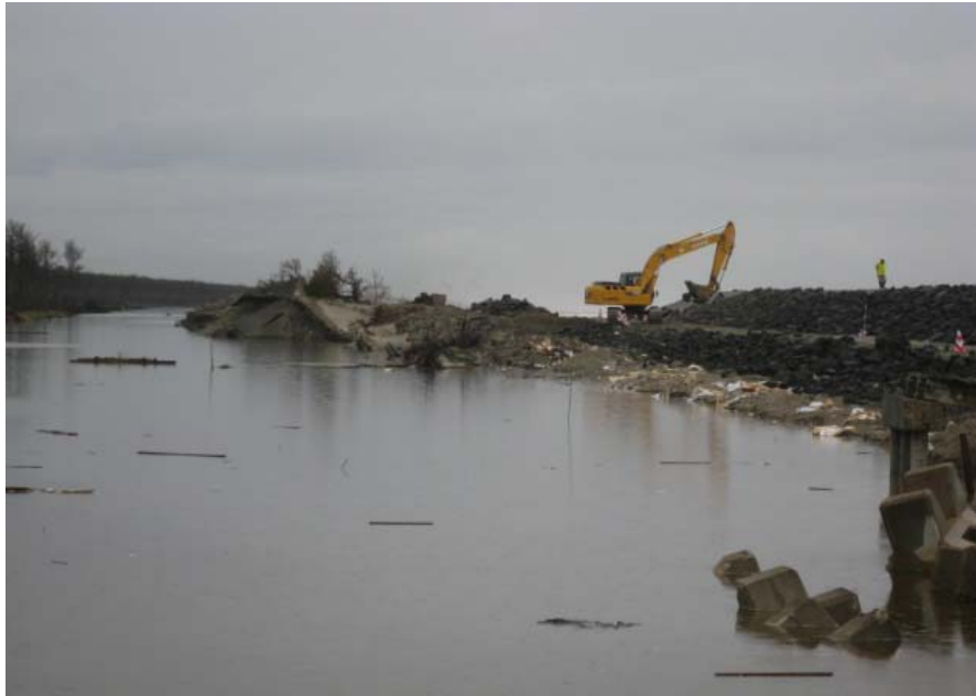
Figure 3.26: Breakage of coastal dike, where the original cross section is displaced several meters inland and its core is exposed due to the lack of a geotextile.
