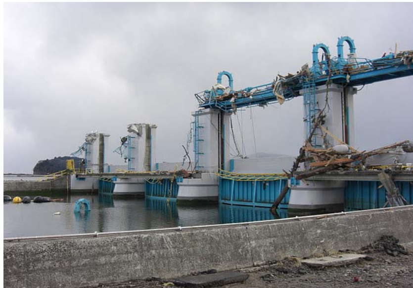
Figure 3.19: Severely damaged storm-surge gates (Source: The 2011 Tohoku Earthquake Tsunami Joint Survey Group; www.coastal.jp/tsunami2011 )
