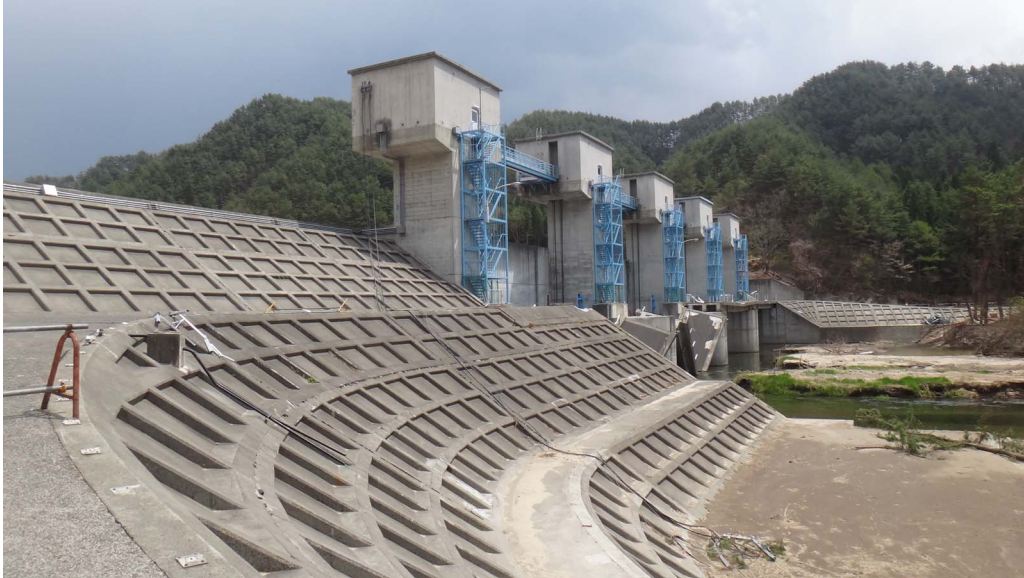
Figure 4.5: Tsunami wall in Fudai (Source: Tokyo University of Marine Science and Technology; courtesy of Akio Okayasu; all rights reserved )
