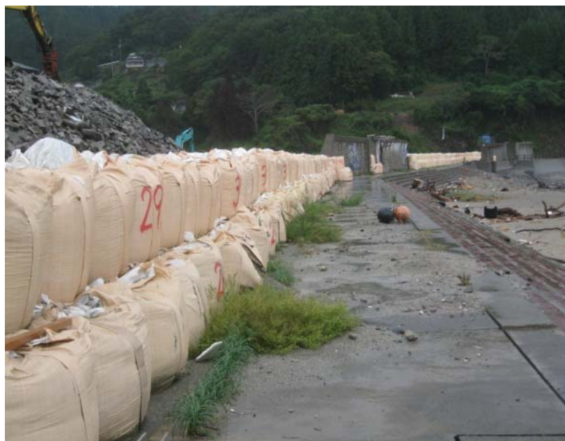
Figure 3.10: Temporary protection measures against storm surges.
