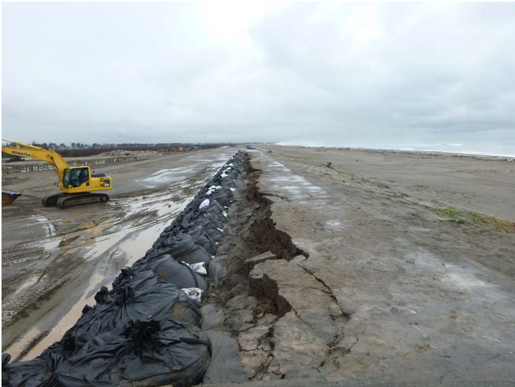
Figure 3.28: Crest of coastal dike one day after the pass of typhoon Roke, 22 September 2011 (Source: Disaster Prevention Research Institute, Kyoto University; Courtesy of Tomohiro Yasuda, all rights reserved )
