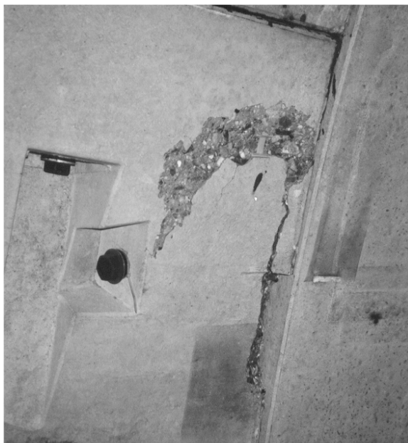
Figure 2 Damage to the Dowel and notch sockets
