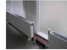
Img 129: Central heating Source: author
