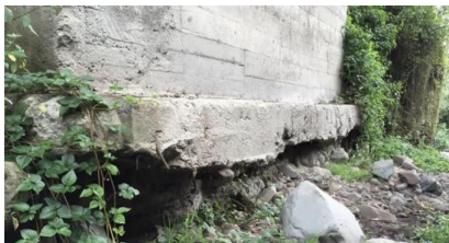
Figure 7. Loss of support contact area in pier C 2014
