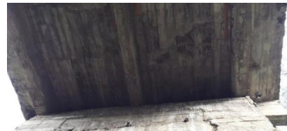
Figure 3. Cracks in the deck of the bridge in 2013
