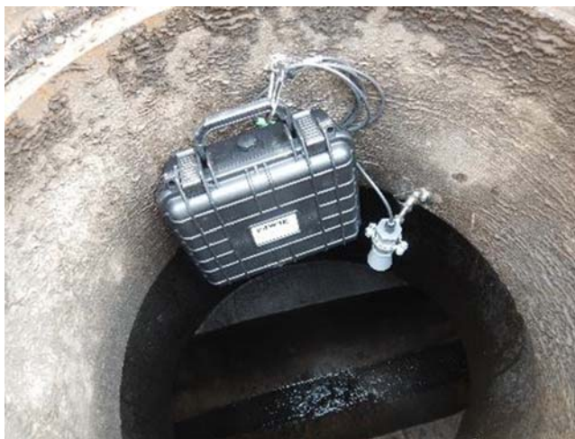
Figure 11.23 LoRaWAN prototype including water level sensor (MaxBotix) installed in a sewer manhole. Source: Eawag.
