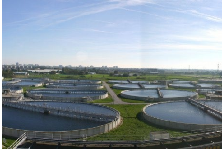
Figure 33 The Harnaschpolder wastewater treatment plant. Delft, The Netherlands.
