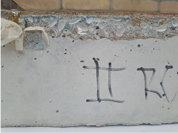
Figure D.13: Close up crack
