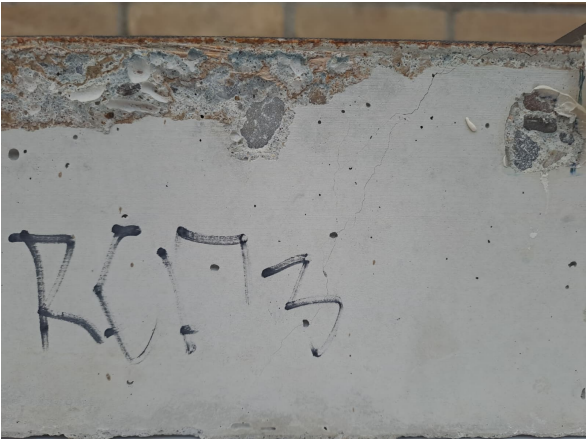
Figure D.14: Close up crack, including crackline along composite
