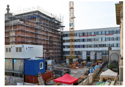
24. Construction site of the bell tower reconstruction. In the background the computer centre. 2020
