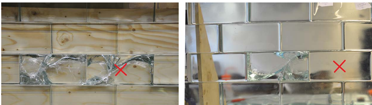
Fig. 15. Left: The prototype before replacement. Right: The prototype after replacement of one of the damaged blocks.
