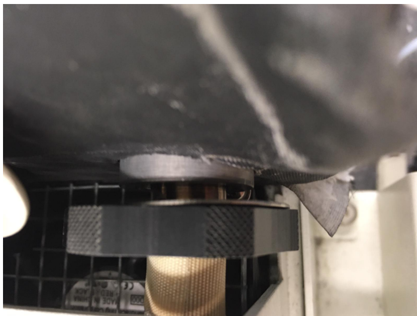
Figure 3.2: A picture of the connection between the first trap and oven.
