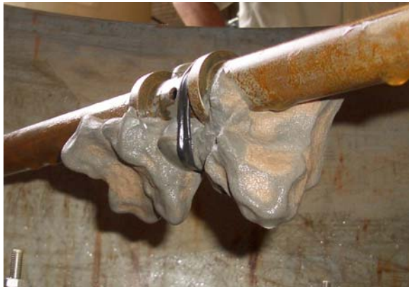
Figure 6-23 Closer picture of the bulb with the rubber sleeve blown up.
