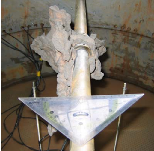
Figure 6-37 Top view of the grout fracture
