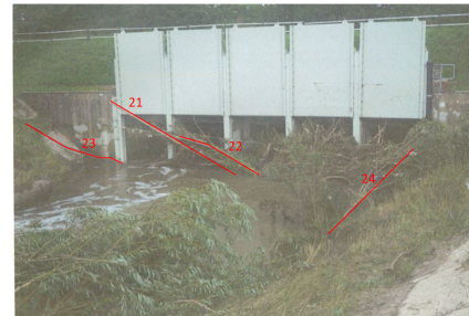
Figure 6.2: Debris after July 2021 event (overview)
