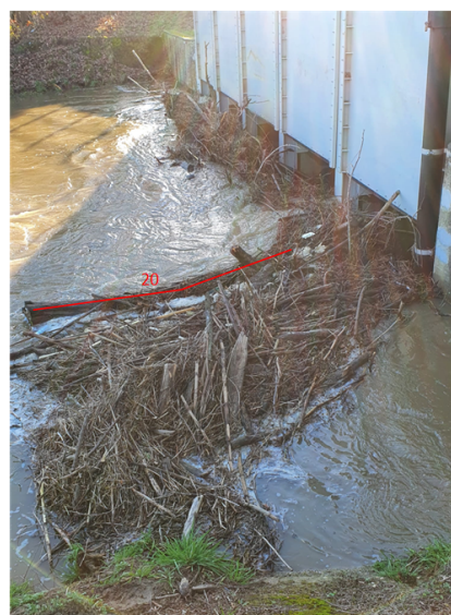
Figure 6.1: Debris during February 2022 event
