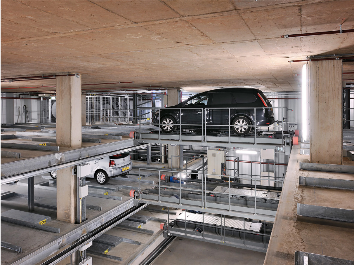
Figure 12: Interior of the parking garage with automated parking system
