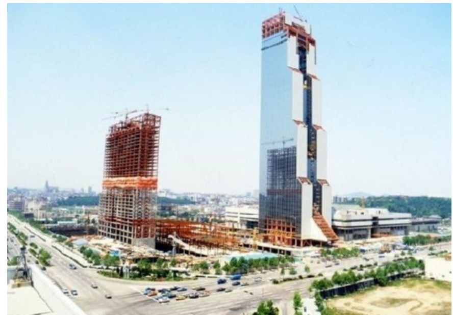
fig.2.8 World Trade Center Seoul in construction 1989 As the Olympics spurred the growth of the Gangnam economy, more modern buildings were raised in the area.
