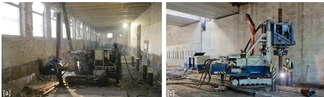
Figure B.36: Examples of pile systems; [a] Internally driven, tubular steel pile; [c] Casing draw pile; (De Waalpaal, 2023).
