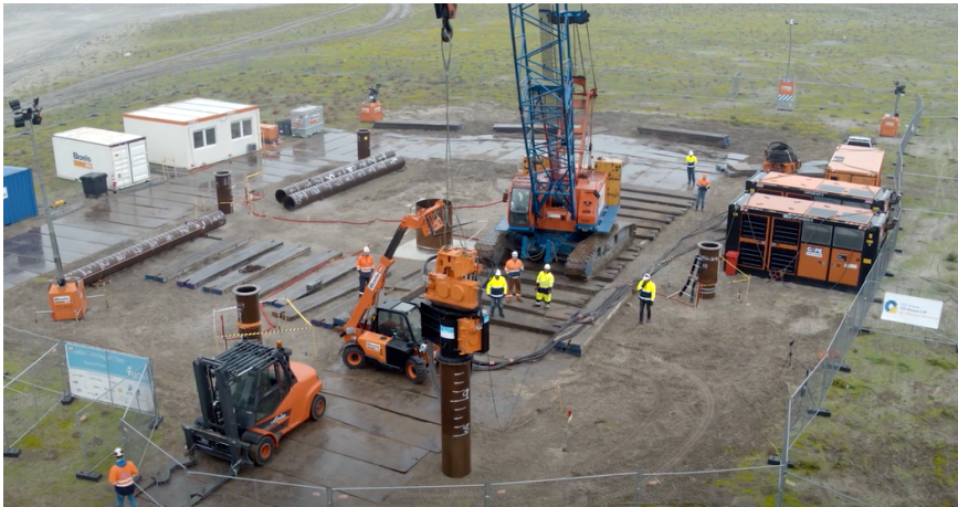
Figure 1.3: The test site of the GDP field campaign at Maasvlakte II in the Port of Rotterdam.
