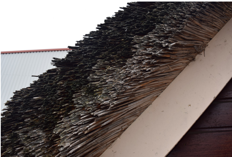
Figure 16: A wet thatch roof in Gouda. It can be seen that the upper layers of reed retain moisture after a period of rain, while the protected lower layers remain dry. (By Author, 2019)
