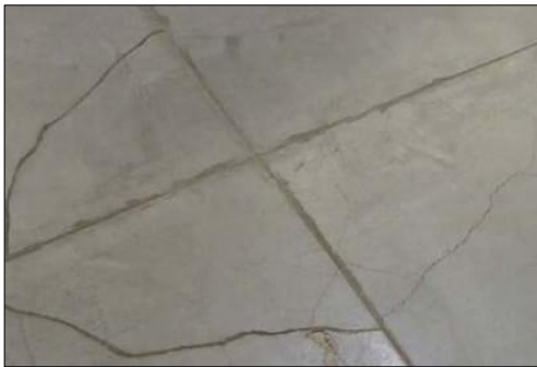
Figure 40. Crack due to curling
