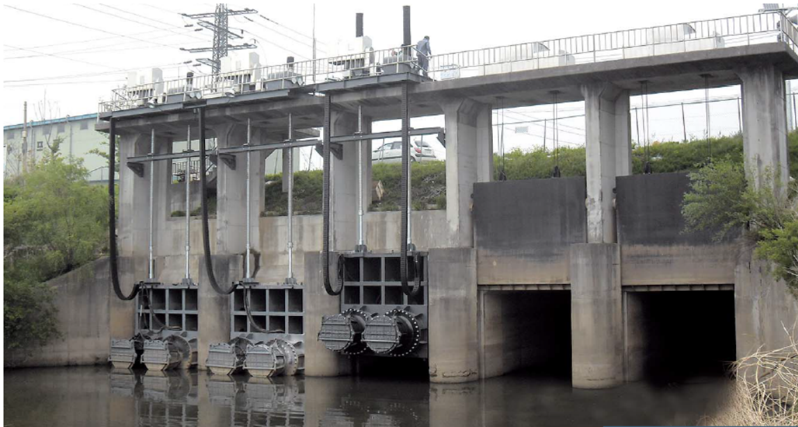
Figure 2.10: Gangmae Pump Station with vertical lifting pump gates
