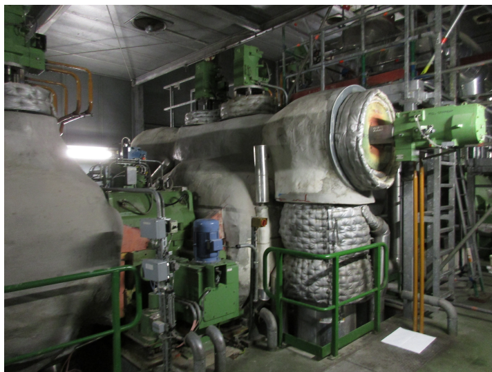
Figure 2.18: View of the MP turbine inlet, with stop valve B (right) and control valves A and B (top)
