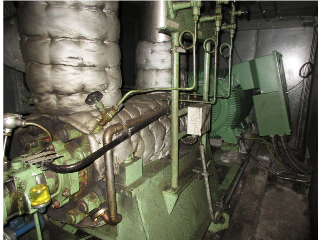
Figure 2.14: View of the HP feedwater pump B
