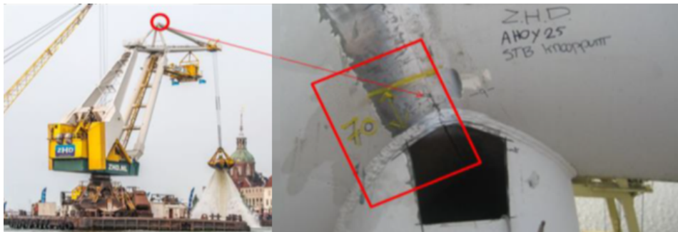
Figure 1.4: Fatigue crack propagation location on Cornelis Tromp 25T Crane [86]
