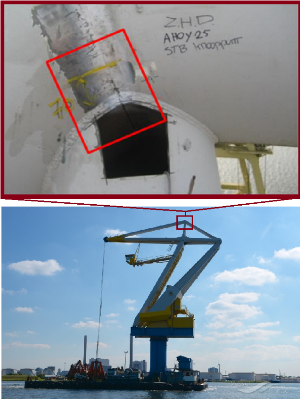
Fig. 1. Crack propagation within upper arm joint of Cornelis Tromp 25T lemniscate crane.
