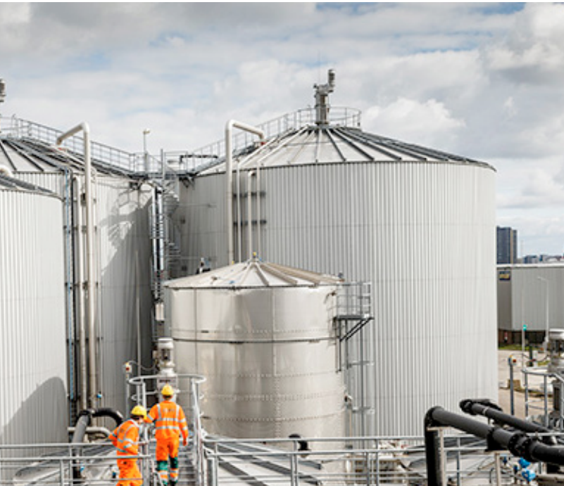
Digesting facility (Orgaworld)
