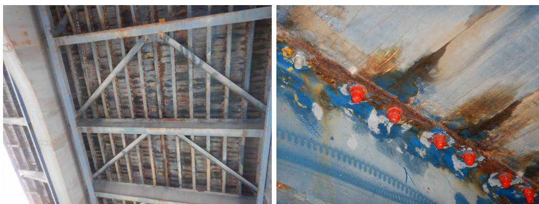
(a) Bottom side of the bascule leaf, showing the degradation of the steel and timber elements (b) Detail of deck-to-longitudinal girder connection in its current state
